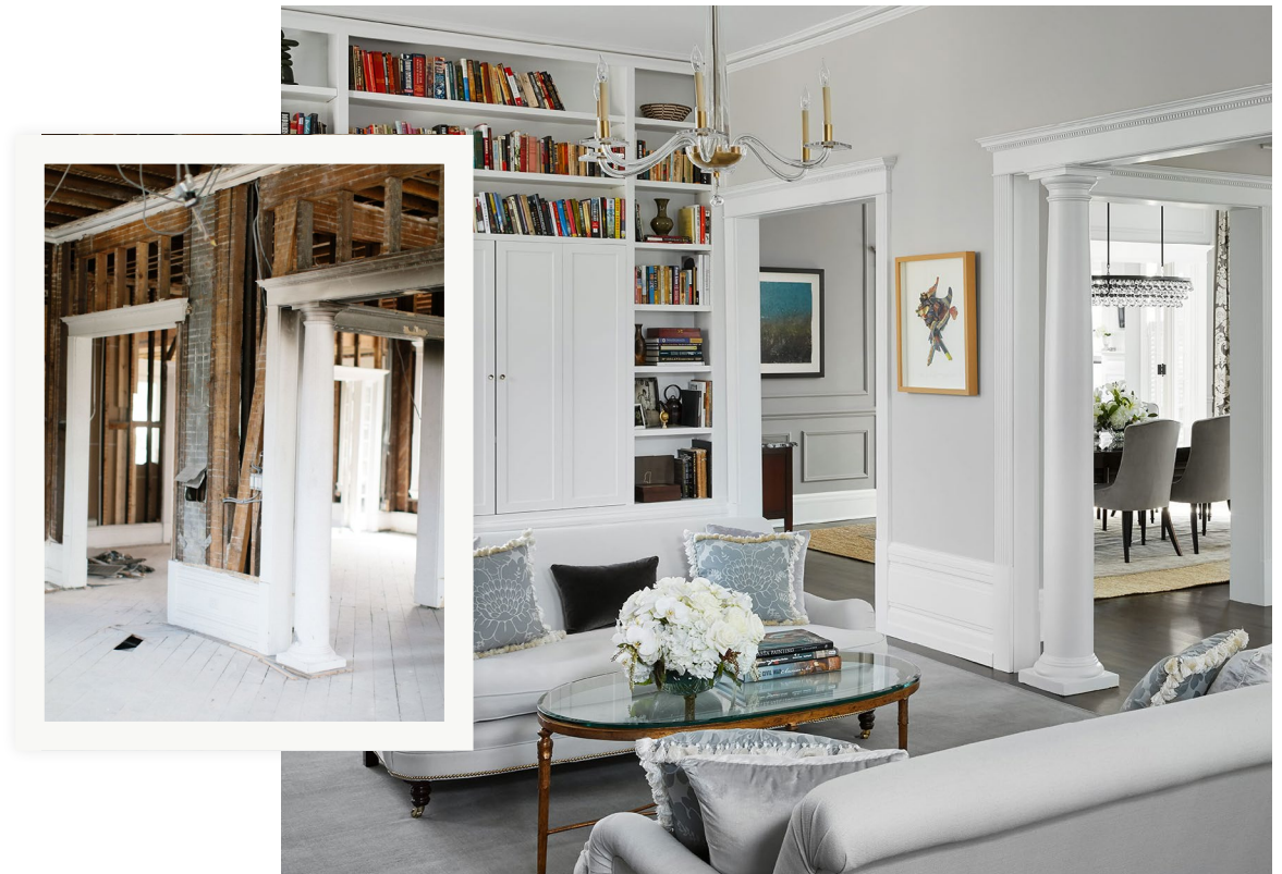
A PURE member's home during and after renovations following a home fire.
